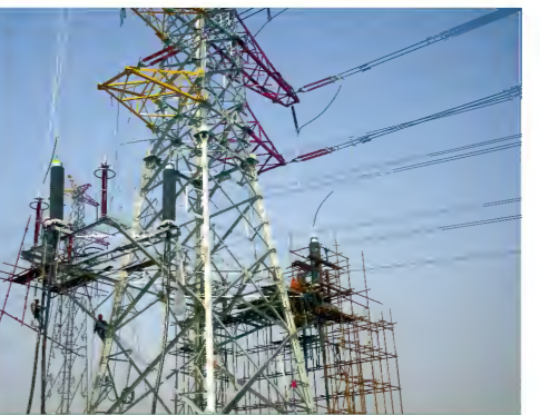
220kV Composite Termination at Changsha Lituo Substation
